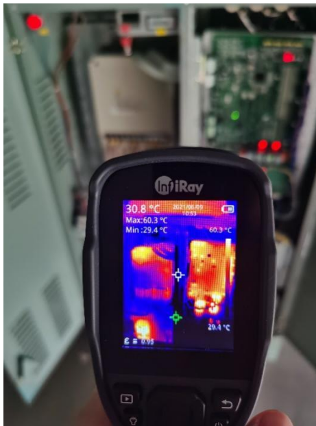
Detecting of Power Distribution Cabinet
